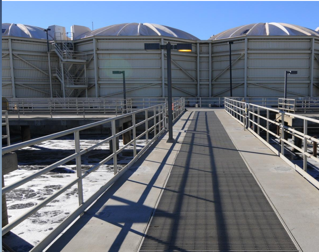
Tower Trickling Filters and Aeration Basins
