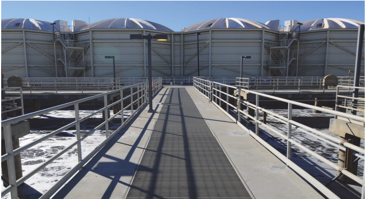
Tower Trickling Filters and Aeration Basins
